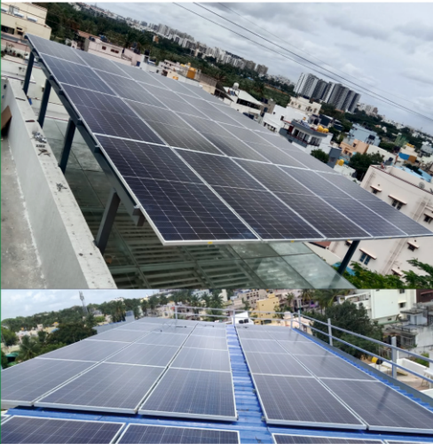
Solar Roof Top
